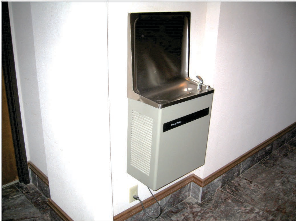
Drinking water coolers
