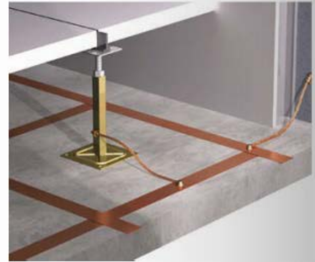
Supplemental bonding grid, or signal reference grid, found in raised-floor systems
